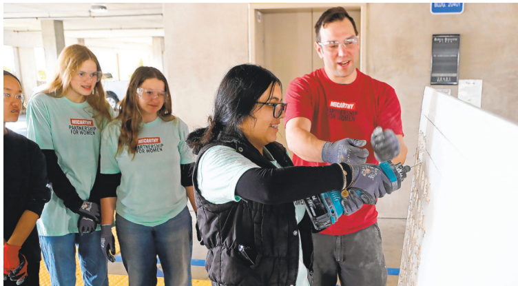
FOREMAN DAVID SANDBROOK encourages Chantal Jimenez, 16, to drill through drywall during McCarthy Building Cos.' Construction 101.
