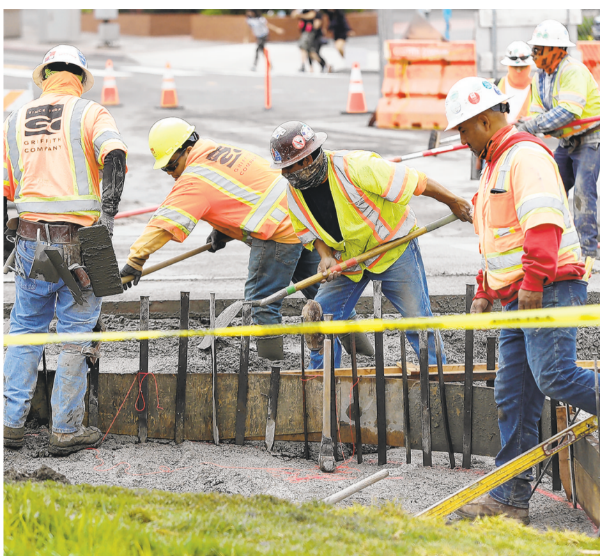
A TEAM OF cement workers pour and fill new cement, making a sidewalk as Caltrans finishes a Laguna Canyon Channel project on Coast Highway in downtown Laguna Beach in May. Preconstruction staging for a sidewalk improvement project along Coast Highway is set to get underway on Tuesday.
