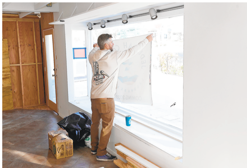
STEVE MUNSEY posts a sign in the space that will be Jedidiah Coffee in North Laguna.
