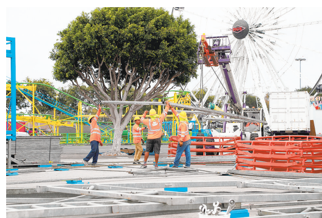
PREPARATIONS FOR the 2021 Orange County Fair, which runs from July 16 through Aug. 15, continued on Tuesday.
