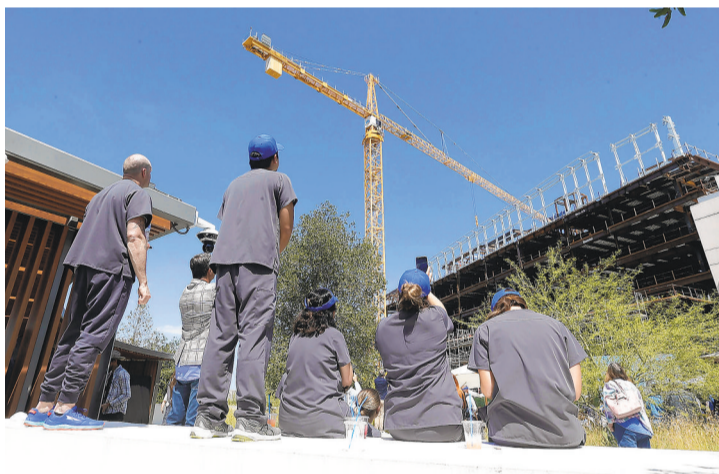
THE FINAL steel beam is lifted by a giant crane onto the coming City of Hope Orange County cancer hospital on Wednesday.
